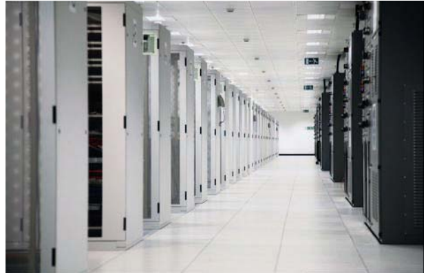
1. Compute farms and data centers drive circuit design innovation due to their need to reduce power consumption.
