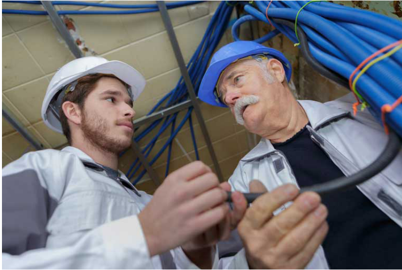
2. The performance of the cabling and interconnects are directly related to the safety of the facility and its operators.
