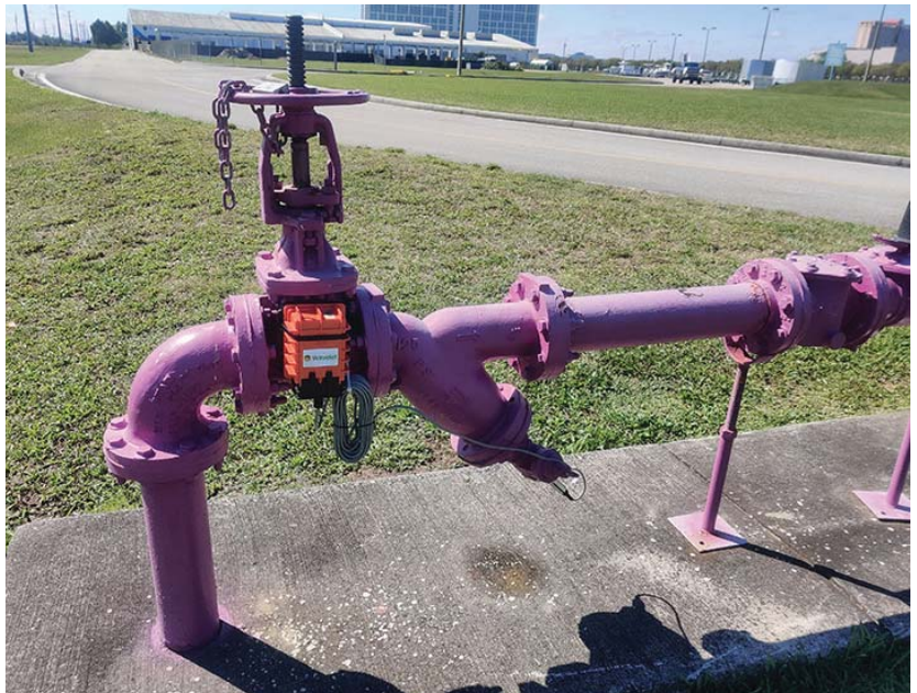
1. Florida's Orange County uses Ayyeka Wavelet devices equipped with Tadiran high-energy LiSOCl 2 batteries to manage the distribution of reclaimed water to golf courses, resorts, and homes.
