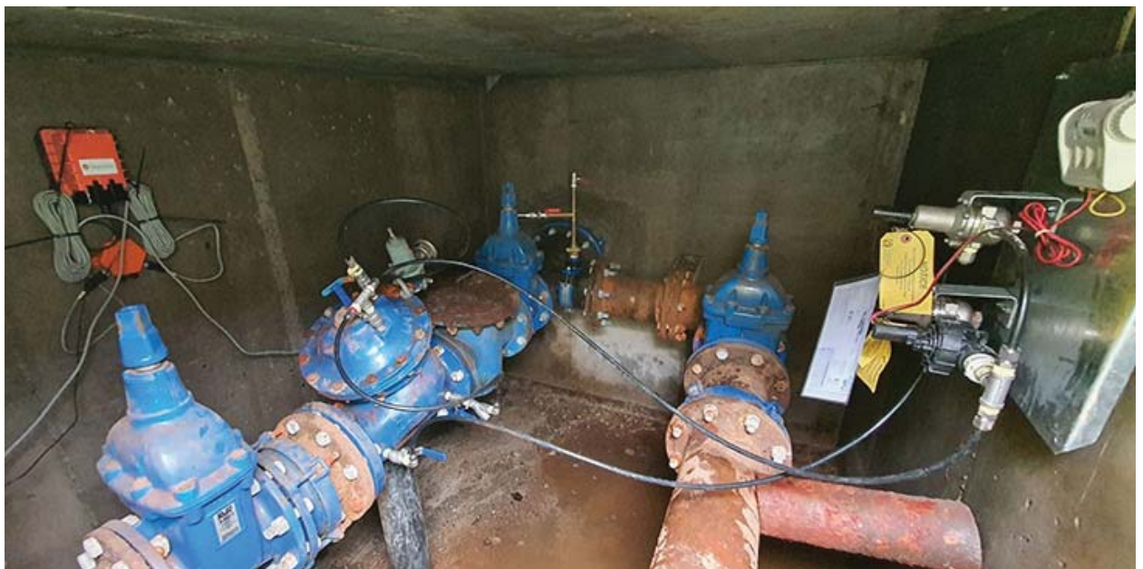
2. Erie County in Pennsylvania uses AI-enabled, battery-powered Wavelet devices to monitor pressure-reducing valves to protect a 100-year-old water system.
